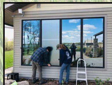
Tyler Dolin and Michala Burke work together to install the anti-collision product on the Visitor Center windows. Photo: Alexa Blankenship/DRWLE-CWMA
