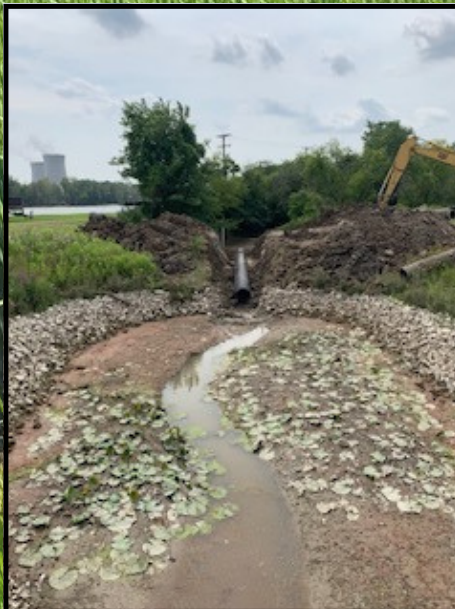
Construction of the pipe and flap gate at Brancheau Unit. Photo: John Nicely/USFWS
