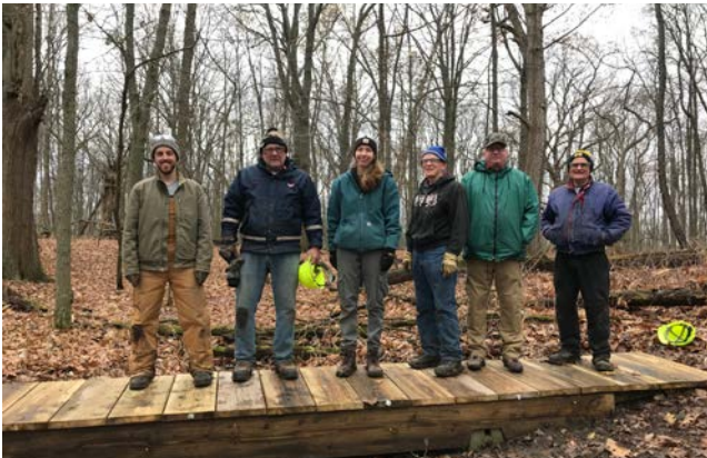
Volunteers braved a cold winter day to build a bridge over an inaccessible portion of the Green Trail. Photo: Six volunteers pose on the new bridge; Jody DeMeyere/USFWS
