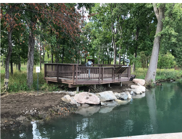
From top: Progress of the shoreline stabilization project at the Humbug observation deck before, during, and after completion. Photos: USFWS
