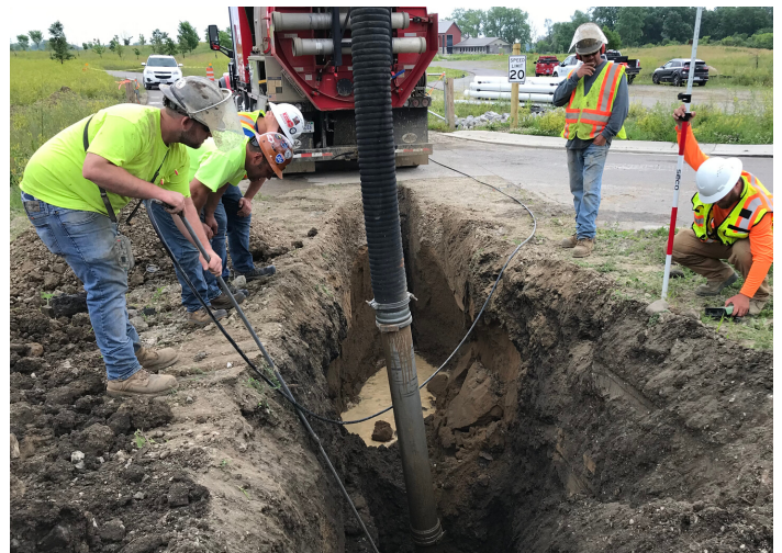
Contractors worked on the sewer lines throughout 2019 and finally fixed the "crap job". Photo: USFWS
