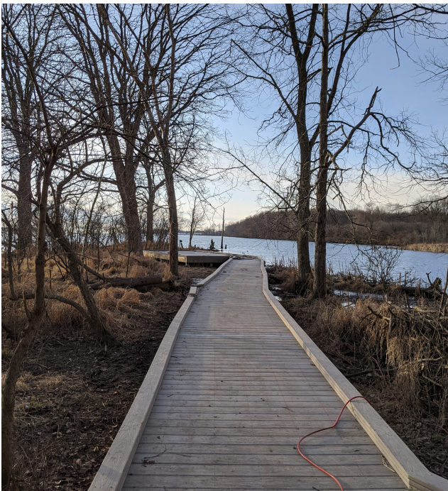
The nearly-completed boardwalk on the Orange Trail at Humbug Marsh. Photo: USFWS
