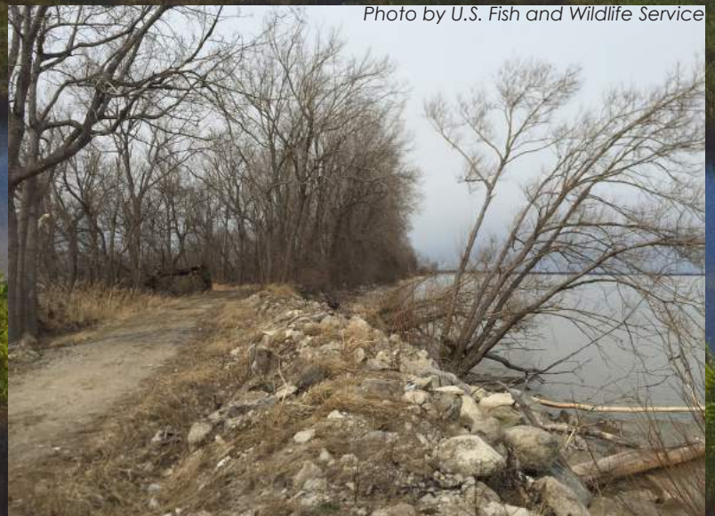
A dike, rebuilt this year, protects Ford Marsh Unit from being flooded by Lake Erie during high water events.
