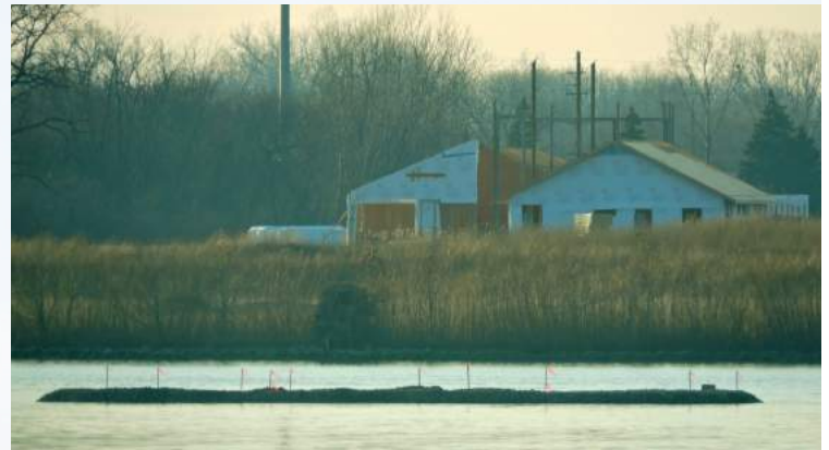
Boat dock and fishing pier construction began in late-2015 with the installation of a stone breakwater in the Detroit River (foreground). The year saw significant progress at the Visitor Center (background).
